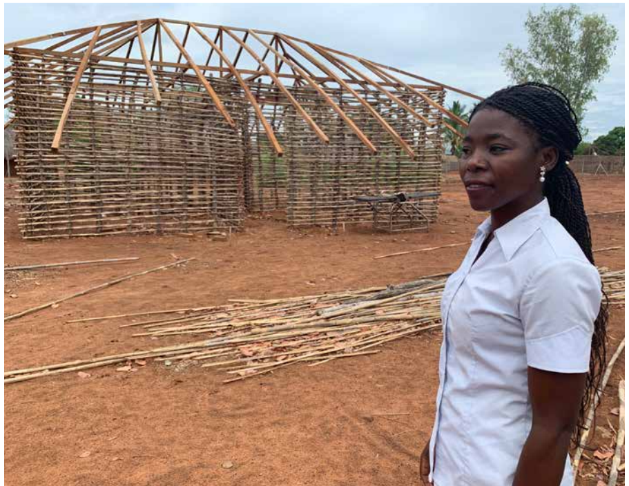
▲ A new mother waiting home being built in Ncumpe. To ensure the pregnant women feel comfortable, it is being built in close collaboration with the villagers. bg
