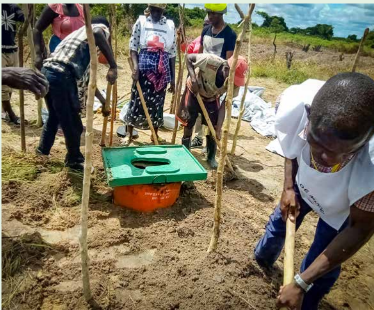
▲ Shortly after the cyclone, SolidarMed's partners set up latrines. Hygiene is crucial to containing the spread of cholera and typhus. Wiwana
