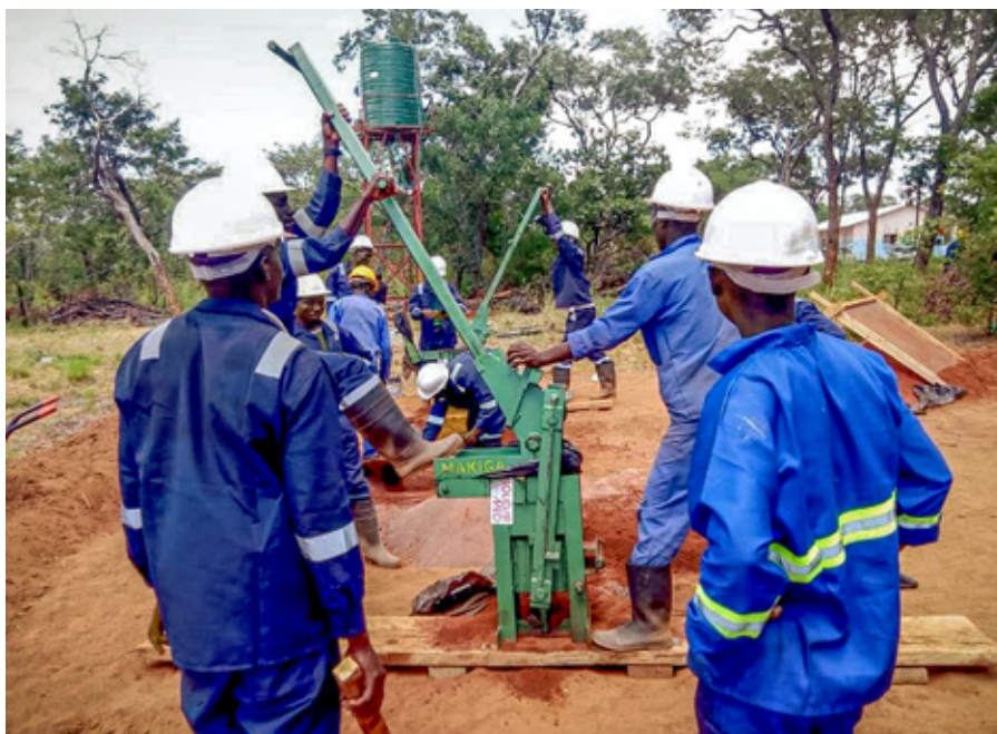
▲ Construction workers forming the blocks made out of soil and cement using the “Makiga” machine. Nzila Lubinda
