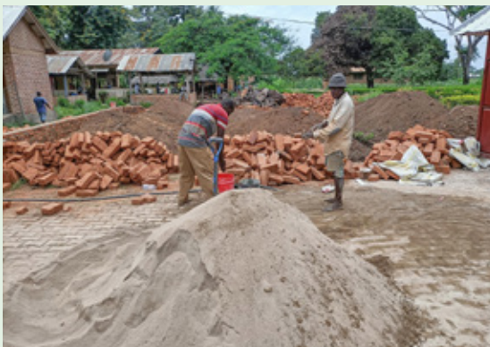
▲ The pharmacy is being built by members of the hospital's own workshop. sm
